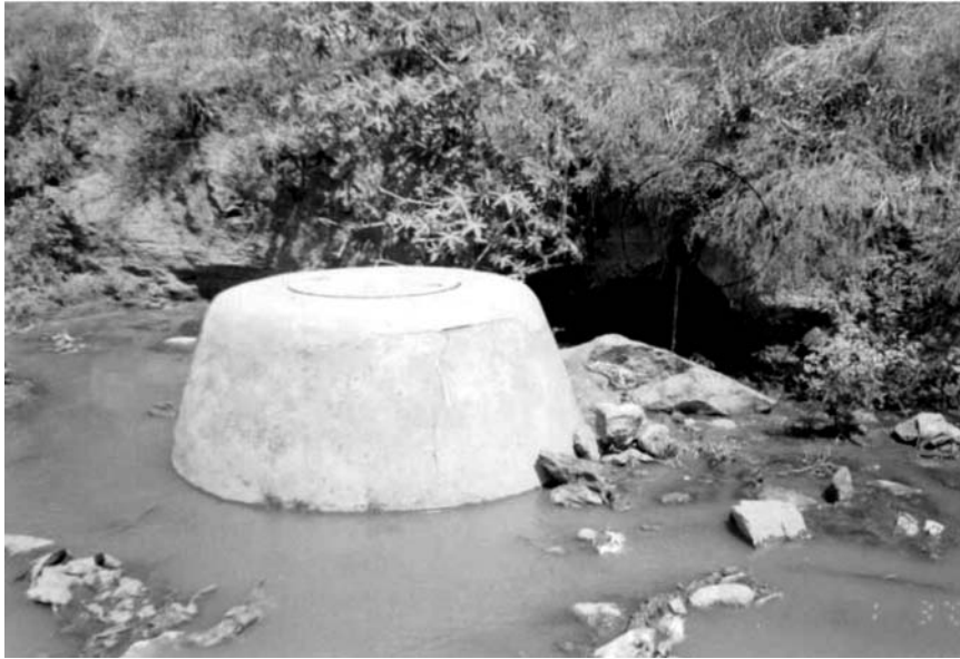
Plate 2.4: Manhole and a sewer connection – obstruction as well as pollution (Source: BWSSB)
